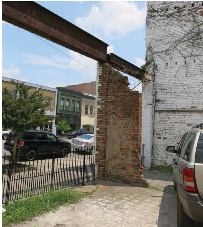
Figure 3.1.18 Existing view from vacant lot proposed for community garden looking out on to Cumberland Avenue.
